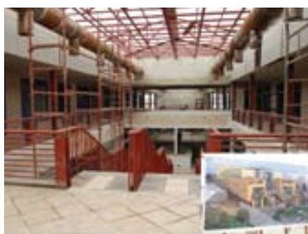
The new Adeniran Ogunsanya Shopping Complex in Surulere, Lagos, under construction with financing from FirstBank
