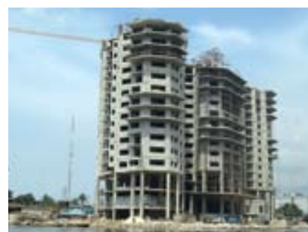
Black Diamond, a residential apartment building under construction in Victoria Island, Lagos owned by Atrib Group, financed by FirstBank
